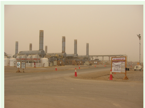
Figure 30-1. Incinerators for solid waste disposal.
